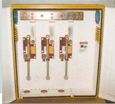
Three 1200 Amp Switches in Fiberglass Cabinet
