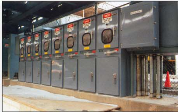
DC Switchgear Lineup Chicago Transit Authority
