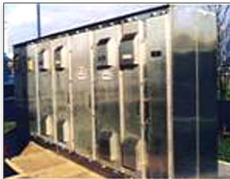
Switch Operator Control Cabinets for Newark Airport Monorail System
